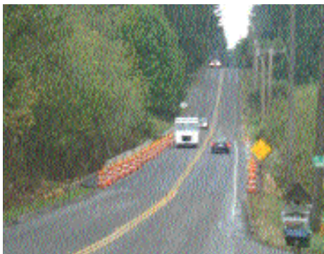
Flooding in a low area of 212th Ave. SE near SE 14 Place should be alleviated now that the roadway has been raised.
