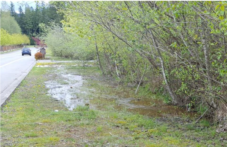
FIGURE 7. FLOODED DITCH ADJACENT TO 248 TH AVE SE.
